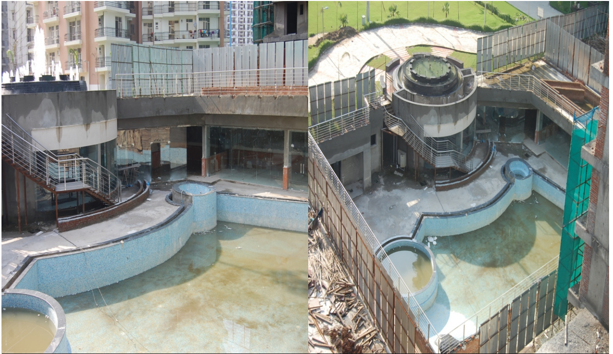
S.K.A Developer Pvt. Ltd., Club Building, Gaur Grandeur Sector-119, NOIDA
